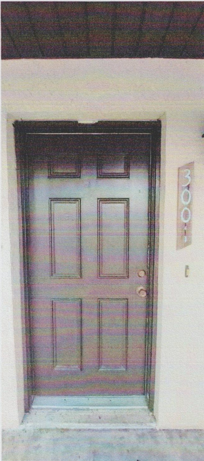
Unprotected non-glazed entry door
