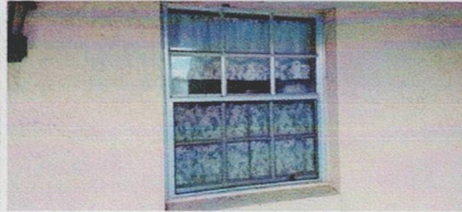
Unprotected glazed opening
